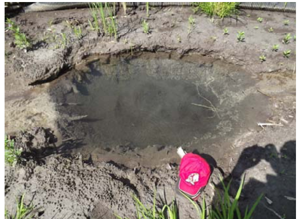
L3/93 corridor sinkhole 8/25/22 credit: Dan Gaither
